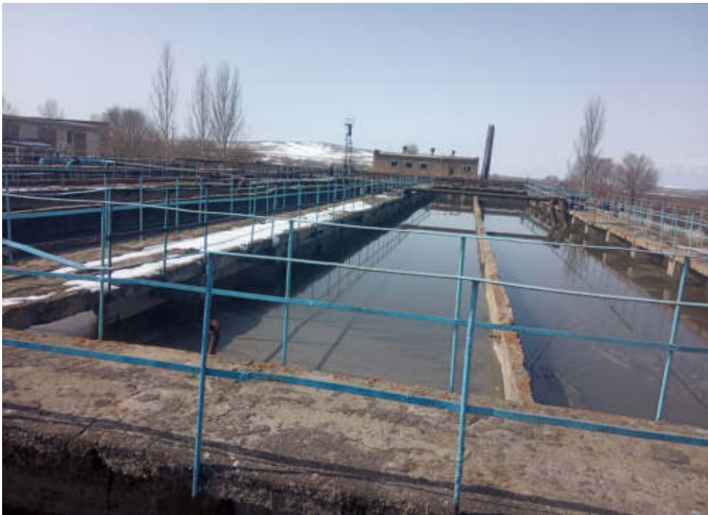
Photo 9. Karakol WWTP. Distribution chamber of pre-sedimentation tank
