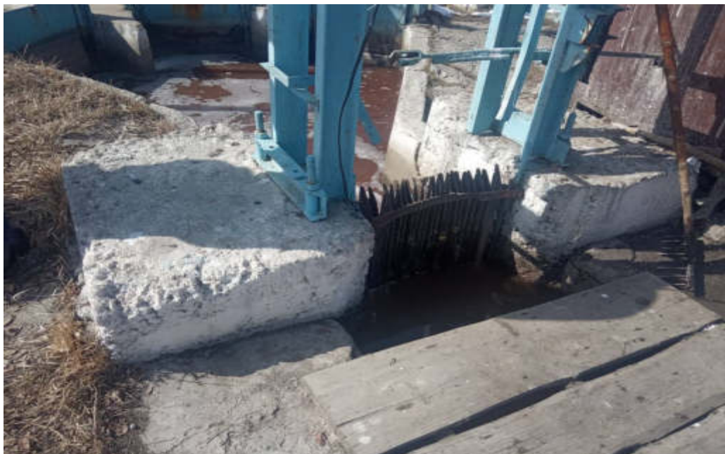
Photo 8. Karakol WWTP. Distribution chamber of pre-sedimentation tank
