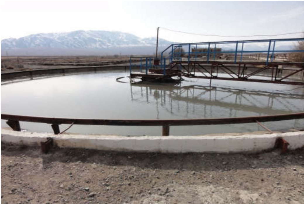
Photo 3. Balykchy WWTP. Pre-sedimentation Tank
