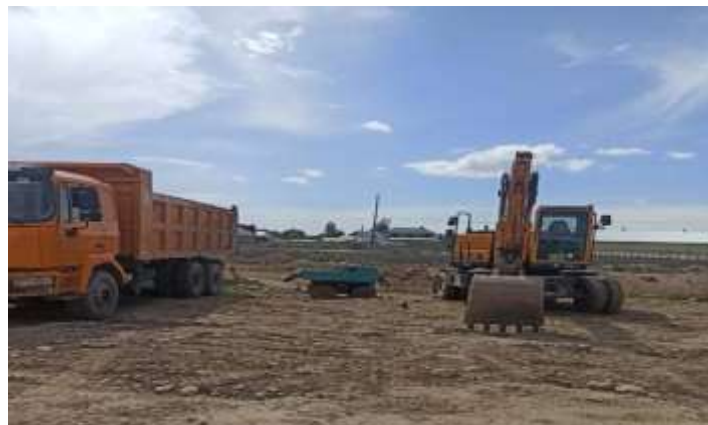
Figure 2-8 Construction site of the consortium of Inzhenernaya Zashchita Ltd. and Polymer Snab Asia Ltd.
