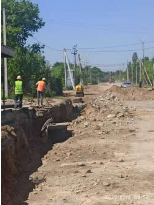
Barricading and display board are not provided in the site
