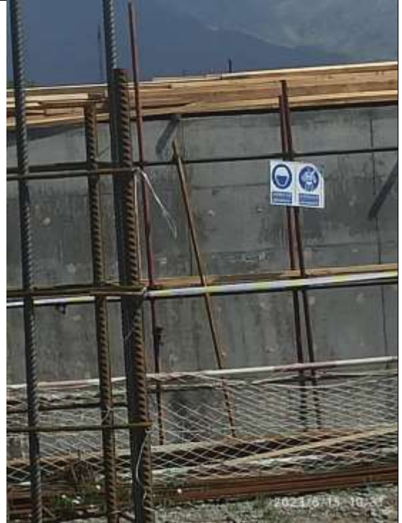
Temporary provision is provided, but the scaffolding is not provided properly
