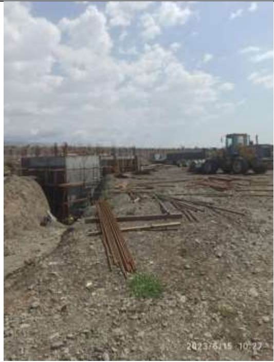
Barricading is not provided, the construction materials are not stored properly
