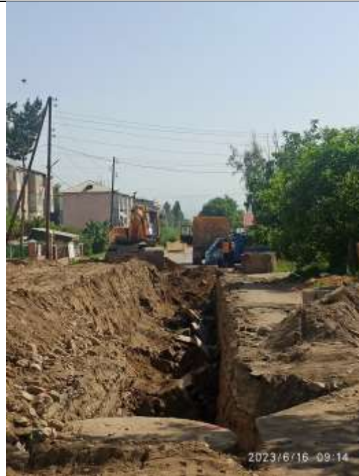
Excess earth has to be removed from the site, temporary passage should have been provided for the locals
