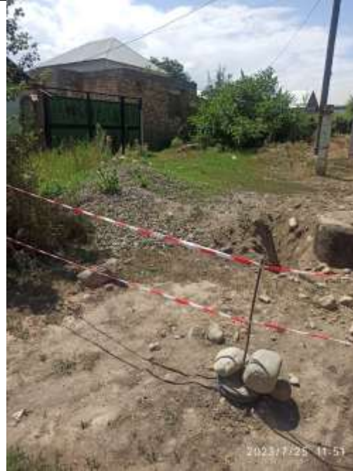
Barricading is observed to be inadequate, it is suggested to provide hard barricading
