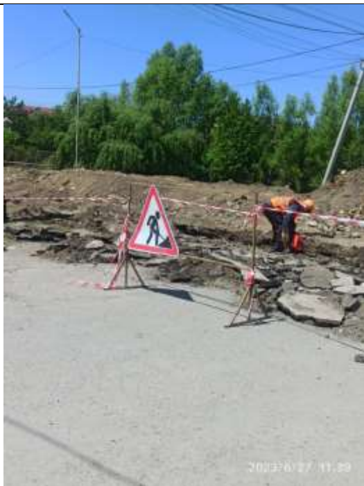
It is suggested to provide hard barricading with solar blinkers for night time road users
