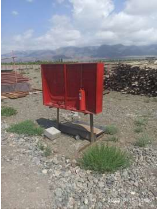
No display boards near the Fire extinguisher
