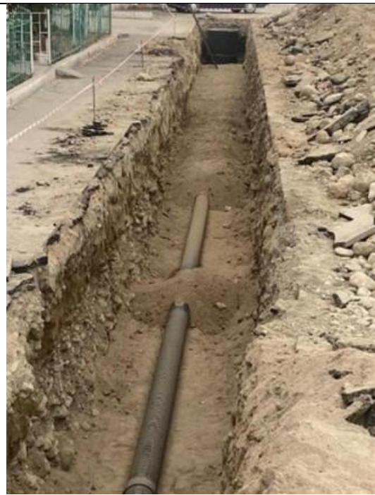
Barricading provided (Safety tape is provided, indicating perimeter control and hazard marking) - Tyupskaya Street
