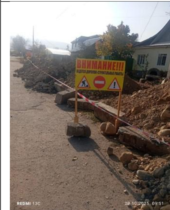
Multilingual hazard signage and - Barricading with red-and-white tape (Effective perimeter control around excavation restricts unauthorized access and reduces fall risk)
