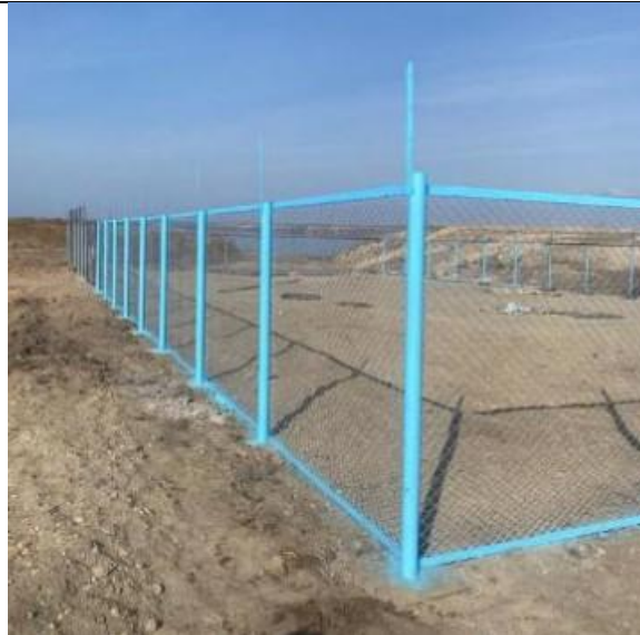
Sewage receiving tank area Buried and Fenced
