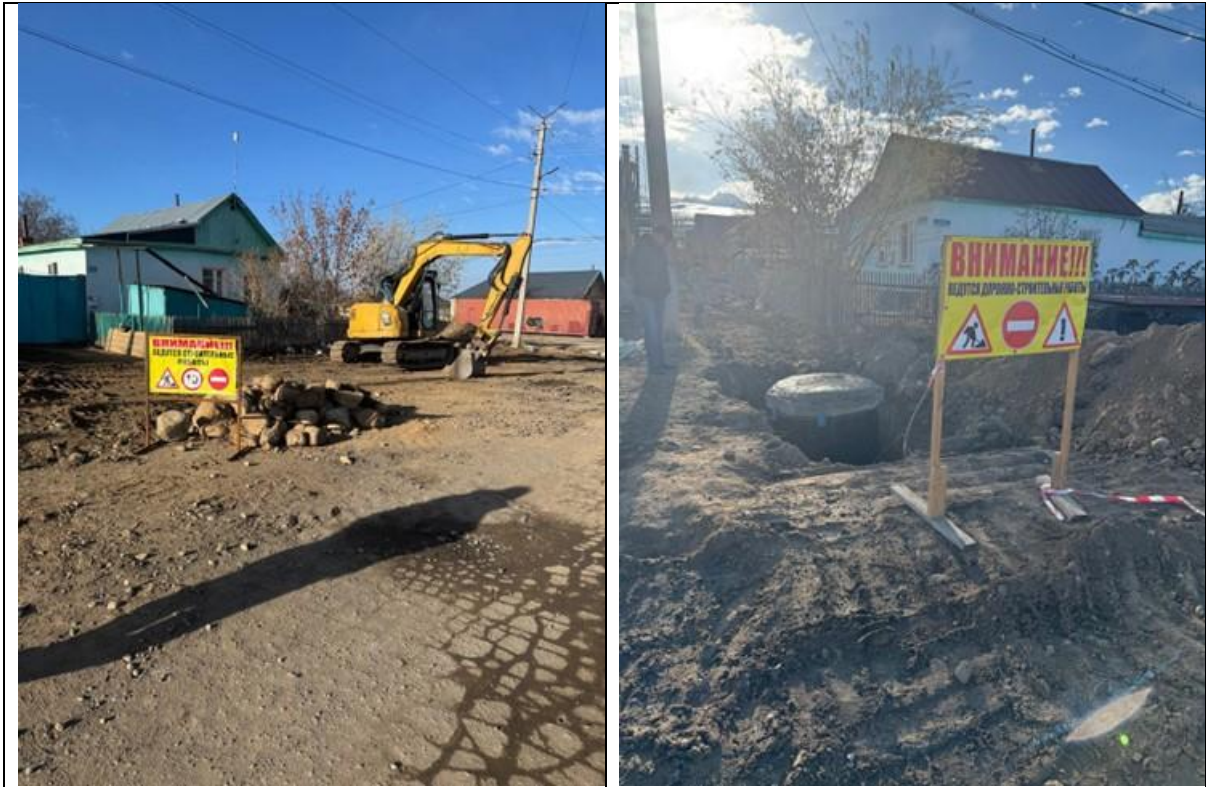
Pipelaying works are in progress on Tupskiy Street and in Geolog Village
