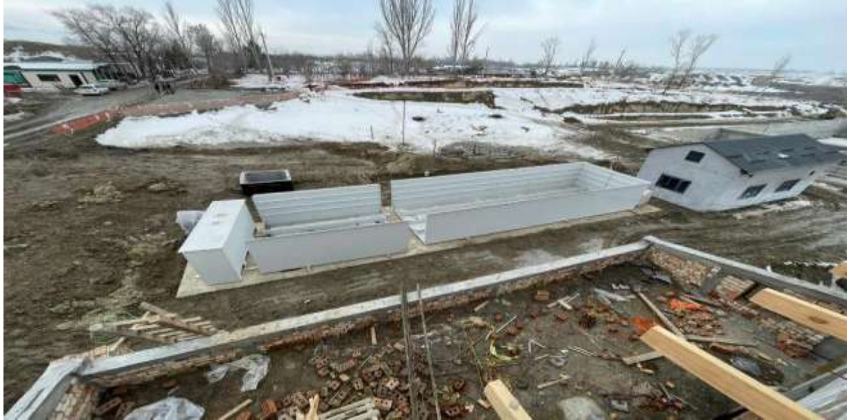
Odor Removal Equipment
