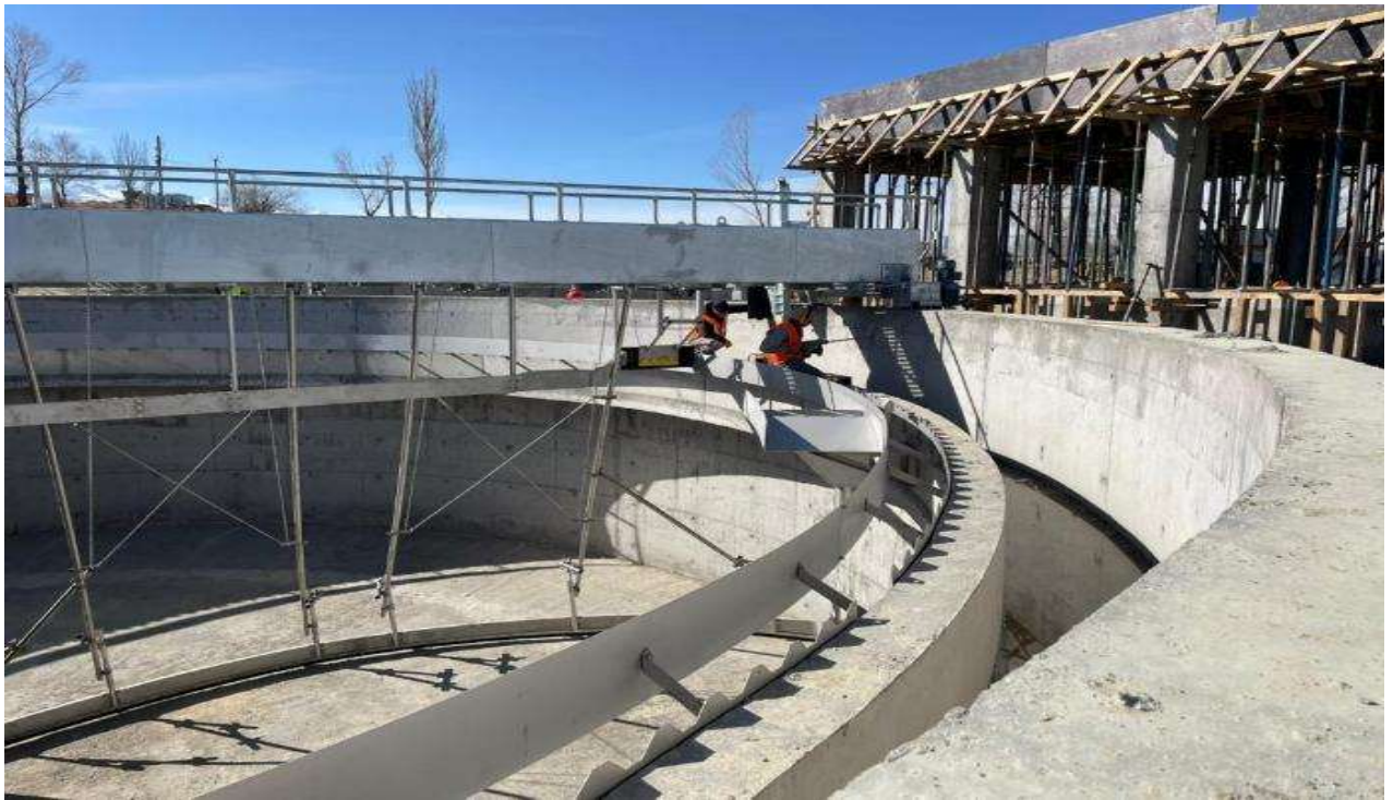
Installed sedimentation tank equipment
